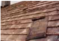
Building structure degradation: mould and mildew
