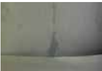
Indoor water damages
