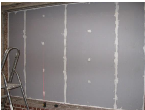
View of Partition from the Source Room
