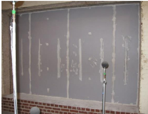
View of Partition from the Source Room
