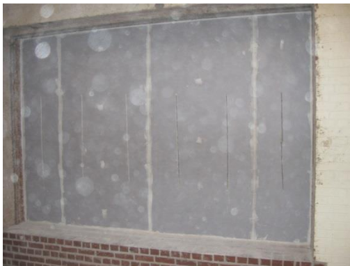
View of Partition from the Source Room
